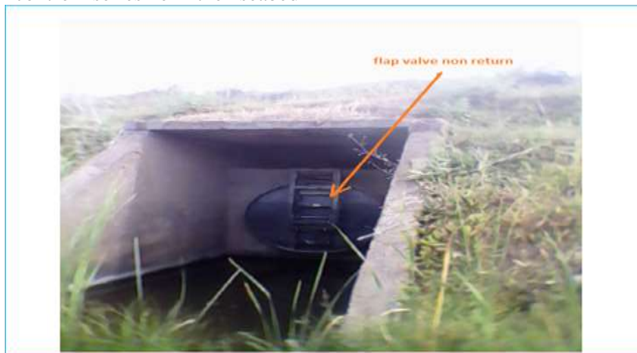
Figure 10. Discharge work under dike leads into El Kebir river canal D03 (photo Sennaoui . F 2016
